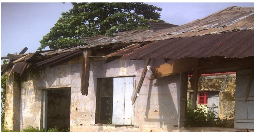
Figure 3: The existing schools in the community are in a state of disrepair Source: Authors' Field Work (2013)
