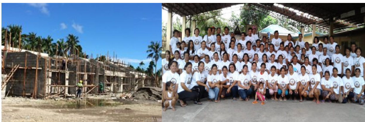
Figure 3b. Ongoing housing construction (Left) and the project beneficiaries (Right) (Photo taken by Gege & Faulmino, 2016)
